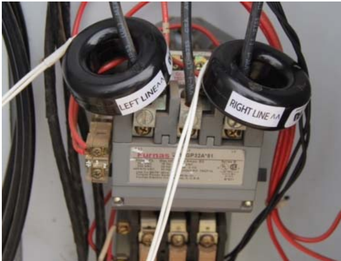
Figure 8 – Current Transformer Installation
