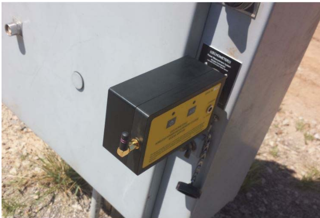
Figure 1 – Installed Wireless Power Sensor
